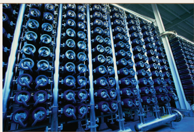
Reverse osmosis cartridge filters as seen in Tampa Bay Seawater Desalination Plant, Tampa, Florida. © David Sailors/Corbis
