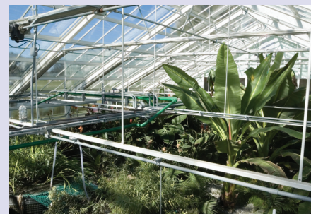
Tropical plants growing inside the greenhouse of the Solar Aquatics Wastewater Treatment have a key role in the water treatment process.
